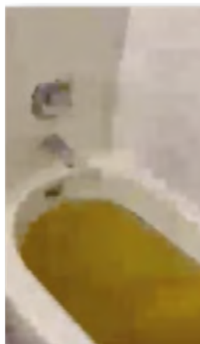
Figure 1: Picture of sewage backflow into the Viera's bathtub less than 24 hours after the family moved into the home.
