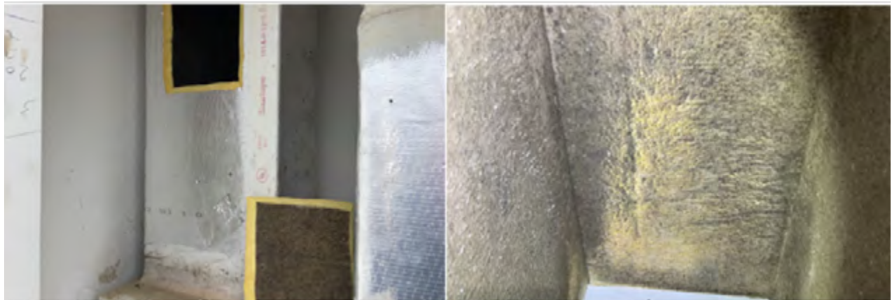
Figure 4: Inside of HVAC system in Erin Greer’s home showing extensive, carpet-like mold growth. 81
