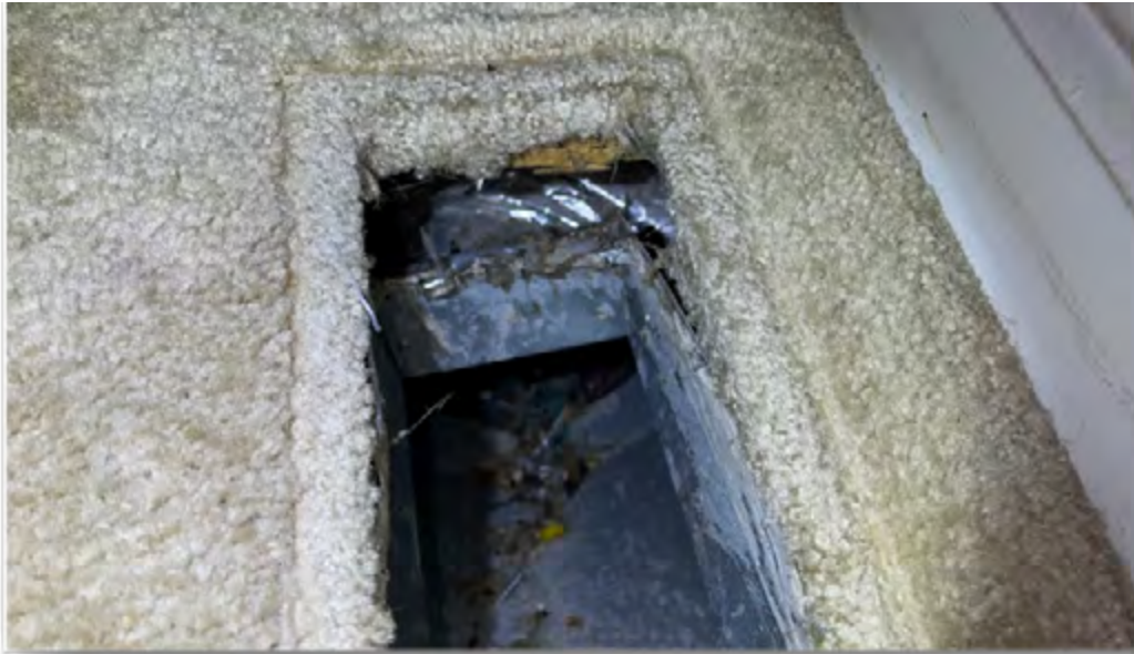
Figure 2: HVAC ducts disconnected from subfloor and from the vents in Erin Greer's home, which potentially exacerbated mold growth. The picture shows the gap between the HVAC metal ducts and the actual vent in the floor. 59
